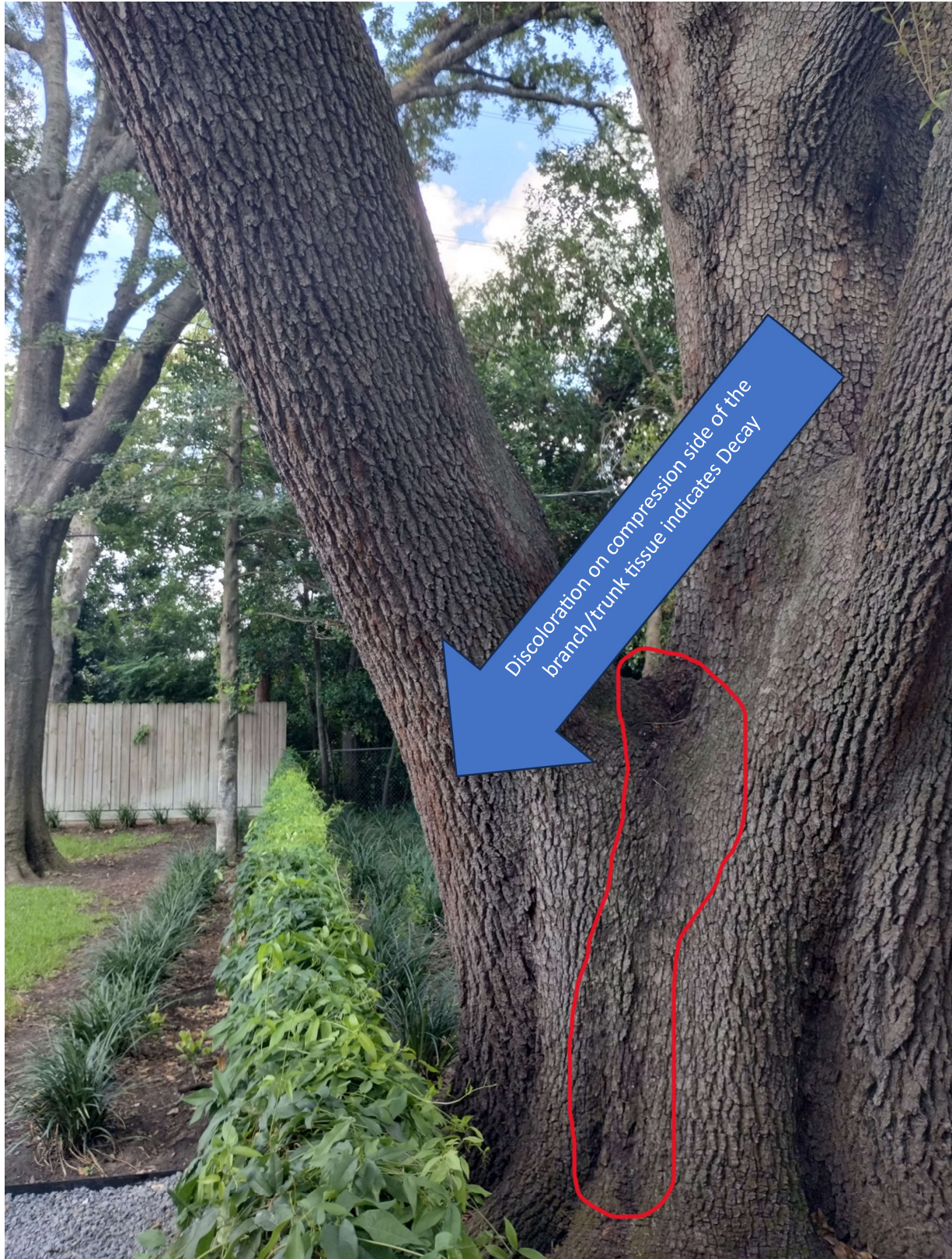
Figure 5 - Base of the Attachment Point of the Limb in question - note the slight cavity and significant crack (branch/Bark Ridge). This is looking opposite the decay point at the base of the limb.
